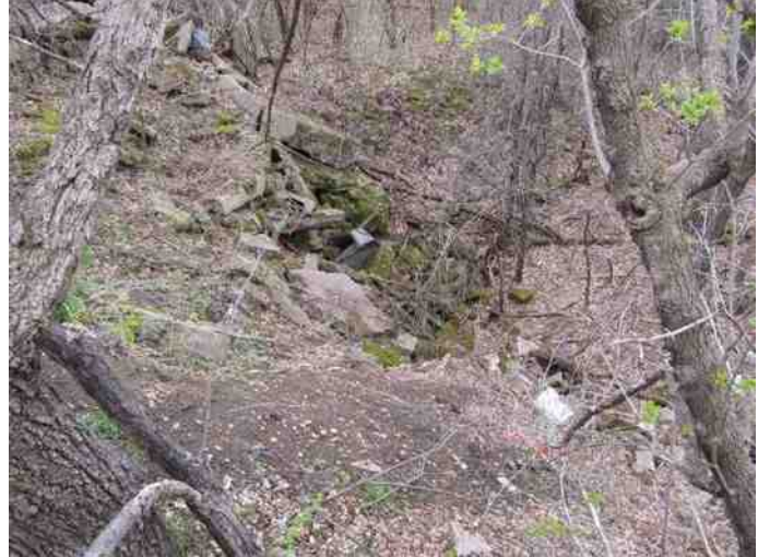
4. DW1 pt13. Debris in east ravine.
